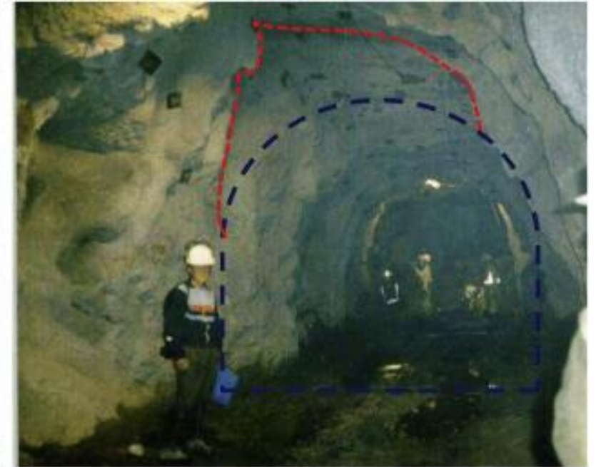
b. Relatively poor quality tunnel contour with excessive over-break (Khimti Project, Nepal)
